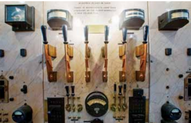
Insulating marble switchboard
